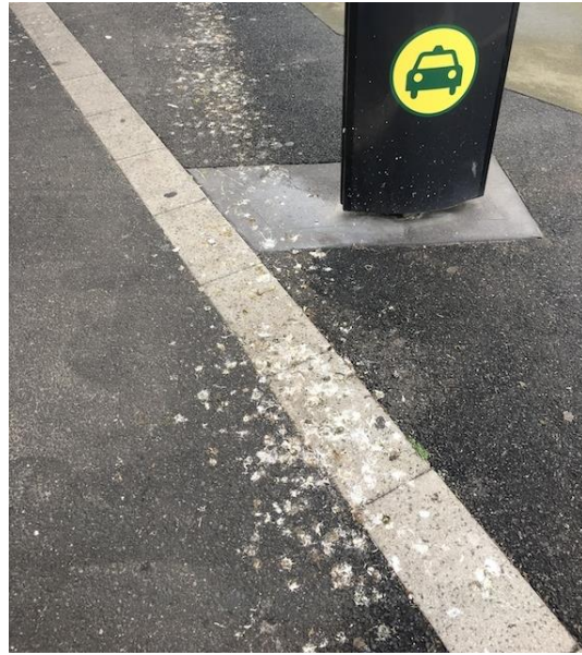
Bird droppings accumulating over time on the footpath (Centre Road East Bentleigh)
