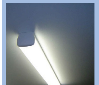
Fluorescent light with shatterproof cover.
