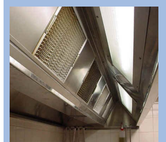
Mechanical exhaust system above cooking appliances.
